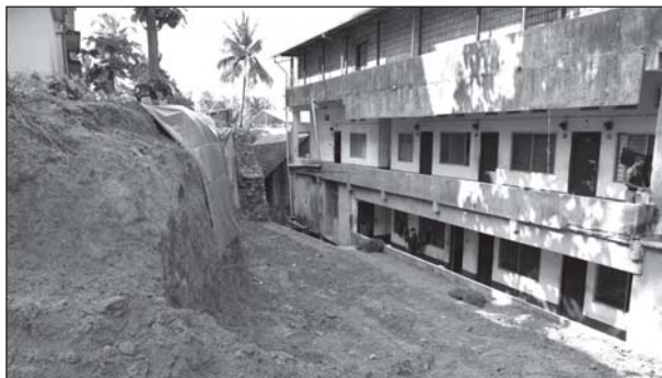
The debris cleared - the Hostel intact!
